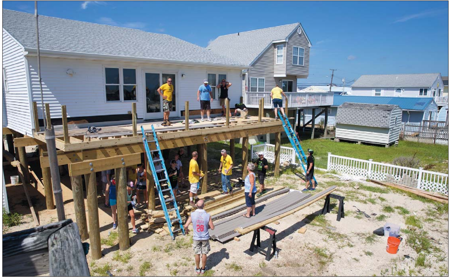
Pictured above: A Future With Hope volunteers help with the rebuilding process of Nan Unley's home in Tuckerton.
