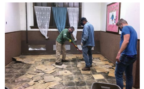
A team of volunteers from Butler UMC participated in a muck-out at Christ Church in Jersey City.
