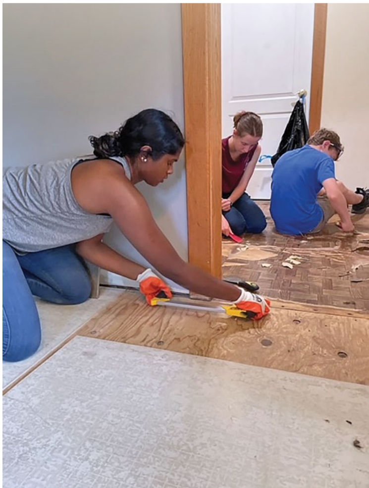
Participants from Sparta UMC, New Dover UMC and Morrow UMC replacing a floor
